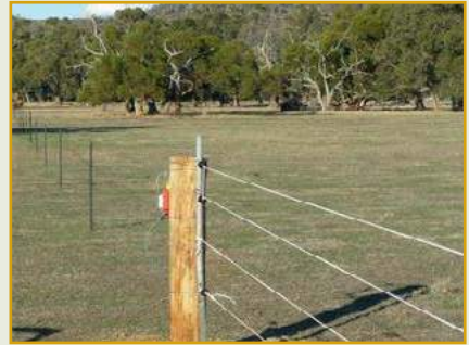
Part of the new fencing installed by Neil to stop access by stock to the vegetated areas (partly funded by the South West Catchment Council).
